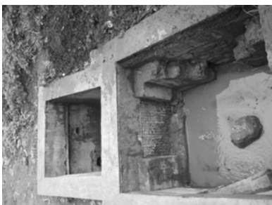
Figure 3: Main exit after degritting
